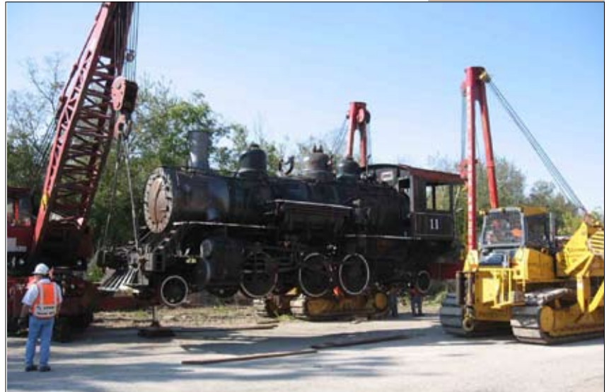
Engine Number 11 hoisted in air prior to being loaded for move to Nicholasville.
