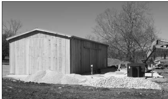
New Nicholasville Sewer Pump Station at 2351 Vince Road across from Carolyn Drive.
